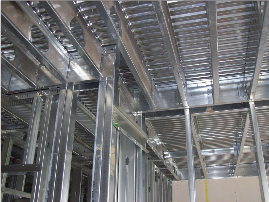
Figure 9-2. Structural systems inspected prior to wall finishes and application of majority of dead load.
