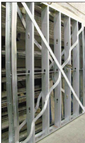
(d) Strap-braced wall after testing, showing yielding in strap (adapted from Comeau 2008 Figure 2.23)
